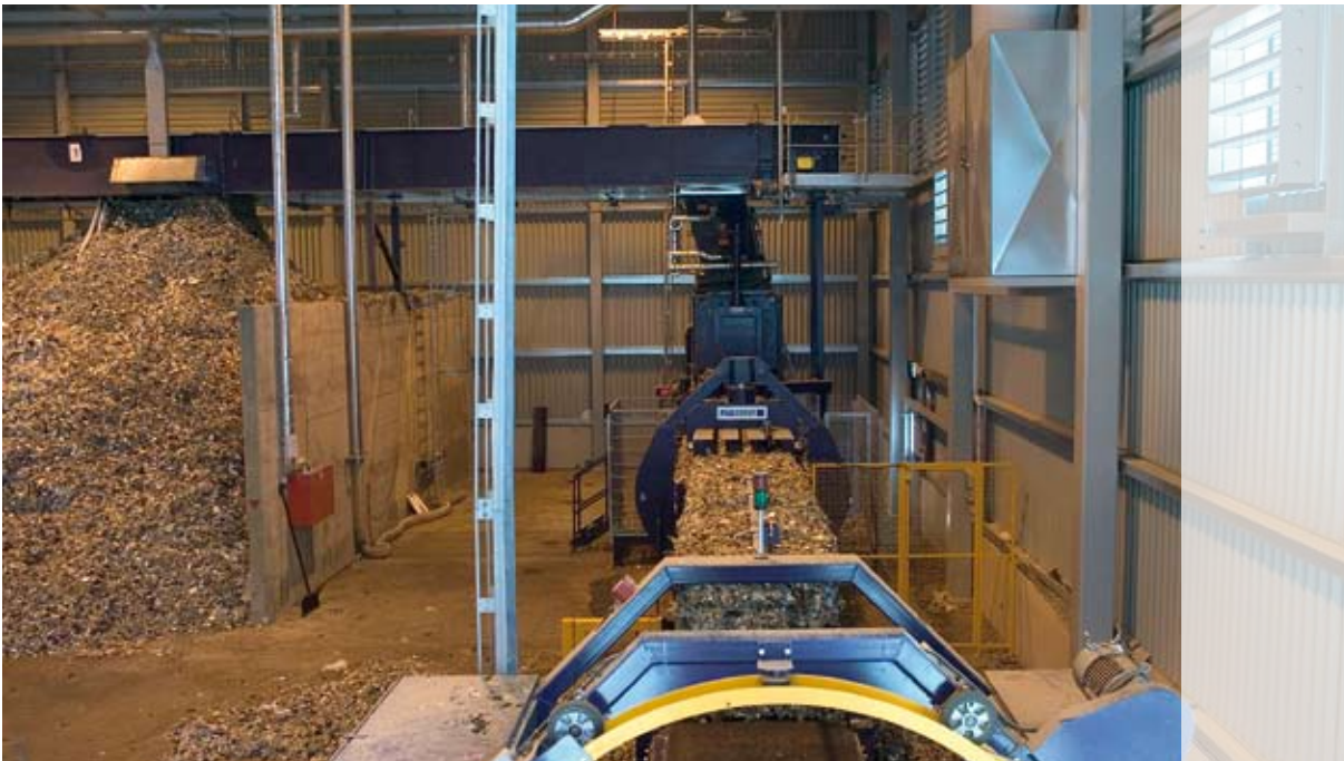
L&T collects burnable waste and processes it into recovered fuel for power plants.
